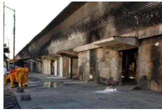
Daños a la Nave Mayor Exterior
