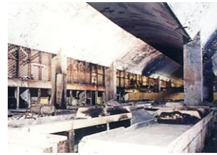
Daños a la Nave Mayor Interior
